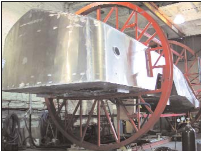
Local 191 members built this huge turning jig to make it easier for welders to reach all areas of the hull. (Photo by Harbour & Shipping Magazine)
