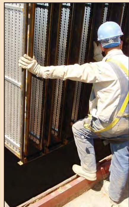
A Boilermaker lines up the agglomerator as it is lowered into its final resting spot, next to a unit's electrostatic precipitator at the Asbury Power Plant.
