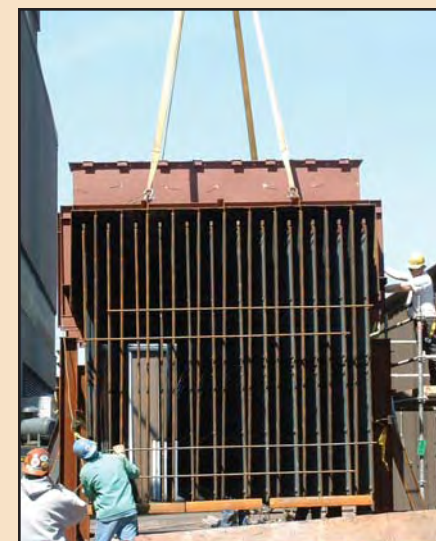
Local 83 members check the rigging before the agglomerator is lifted into place.
